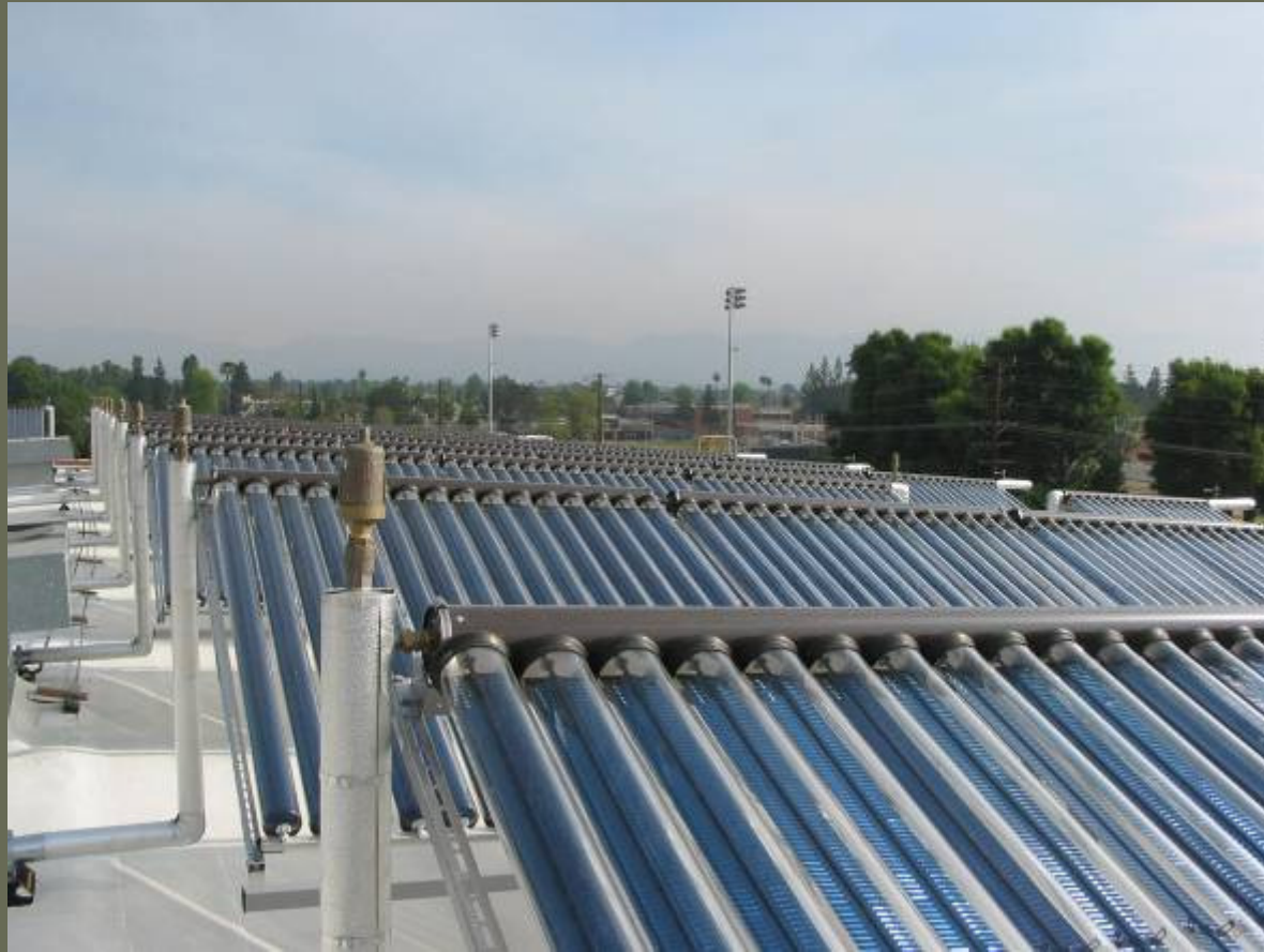
North Gym Solar Water Heating Panels
